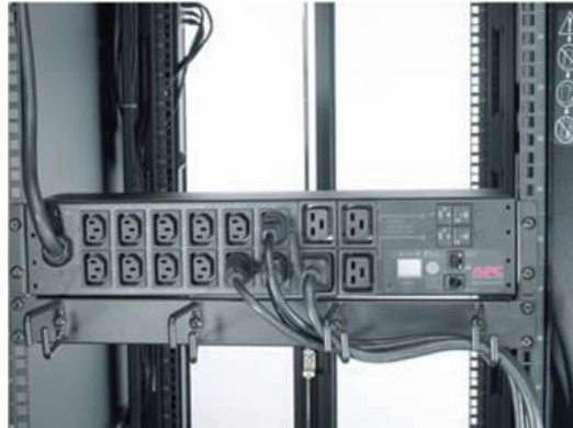
3.2.4: Power Distribution Unit [10]
